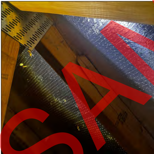
Cracked truss member near garage attic access entrance. PHOTO A
