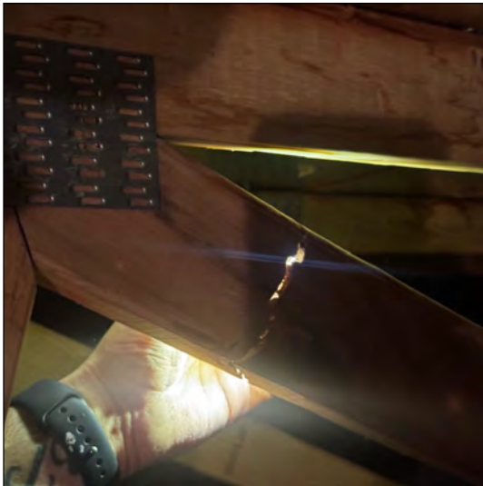
Cracked truss member near air handler platform. PHOTO A
