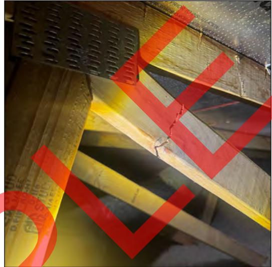
Cracked truss member near air handler platform. PHOTO B
