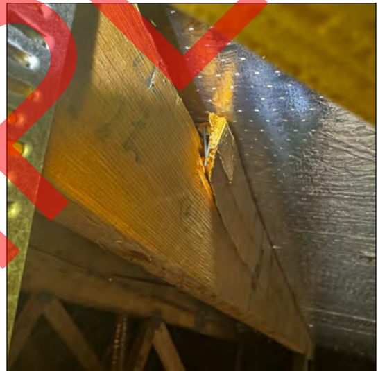
Cracked truss member near garage attic access entrance. PHOTO B
